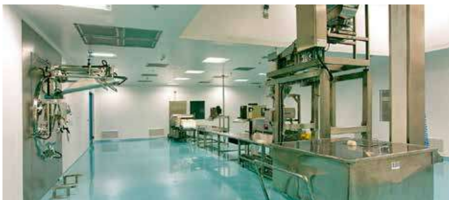
Figure 3: In state-of-the-art plants, products are manufactured under cleanroom conditions.
